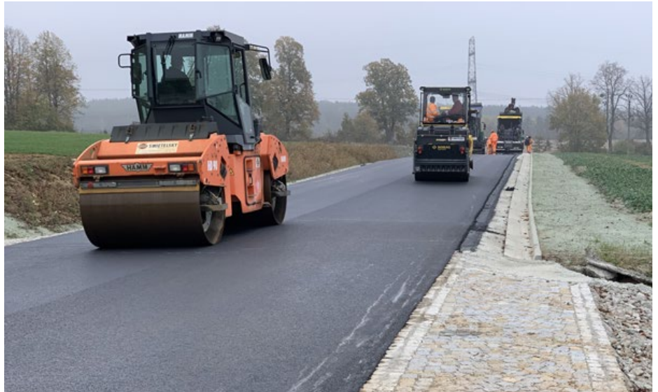
Public road, privately built: With the 2 km long bypass road, Kámen a písek contributes to the common good and to an increase in the quality of life of the village residents.
