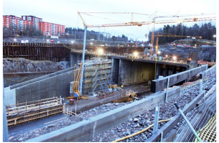
E4 Stockholm Bypass: The 3 bn USD project is one of the largest and most complex in the history of road construction in Sweden and will feature a 16.5-km tunnel, which goes under Mälaren lake at a depth of 100 metres.
