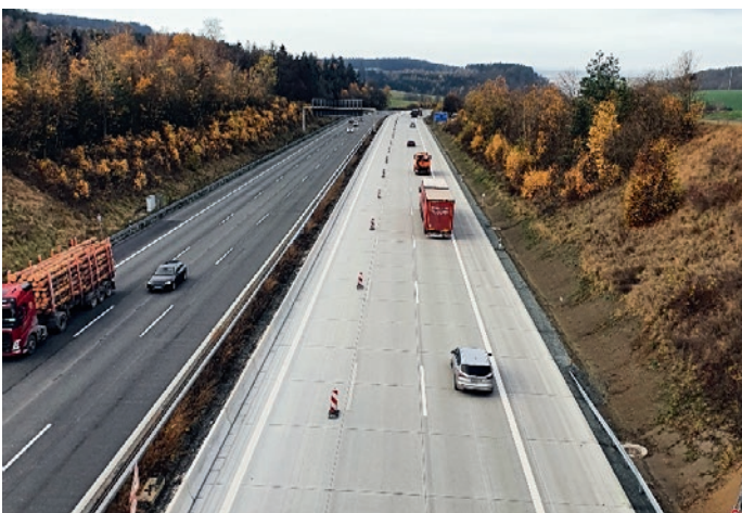
The company's own installation team with seven experienced installers is in demand for projects such as the one on the A9 near Marktschorgast, in order to cope with the complexity of permanent installation projects.
