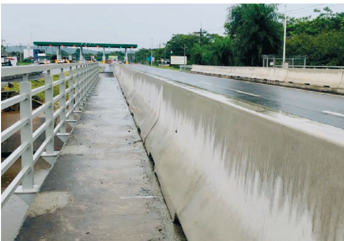
Megaproject in Paraguay: 113 km (!) of Deltabloc® elements have been installed along the Rota del Este towards Brazil since 2018.
